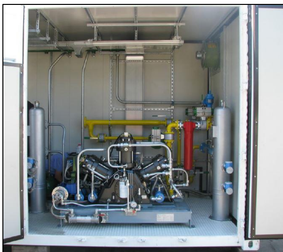
Figure 2: Biomethane compression unit
