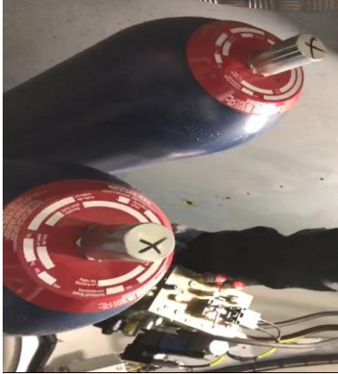
Figure 3. Picture of two bladder hydraulic accumulators installed inside the nacelle of a wind turbine of the Mazara del Vallo wind farm (province of Trapani), made by the authors.
