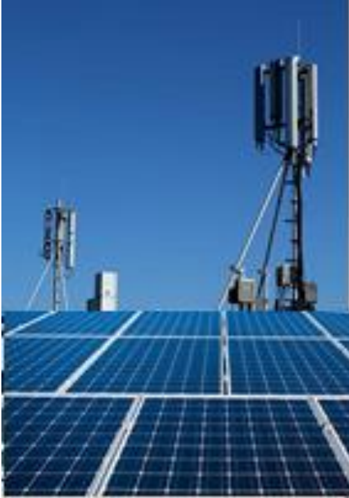
Figure 1: A 4G antenna, built near a small photovoltaic system installed on the roof of a building.
