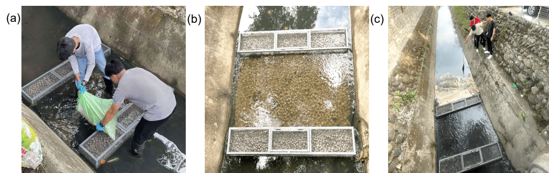
Figure 2: (a) Field application of gabion mattress, (b) installed prototype, and (c) in-situ water quality monitoring using Horiba Multi-Parameter Meter
